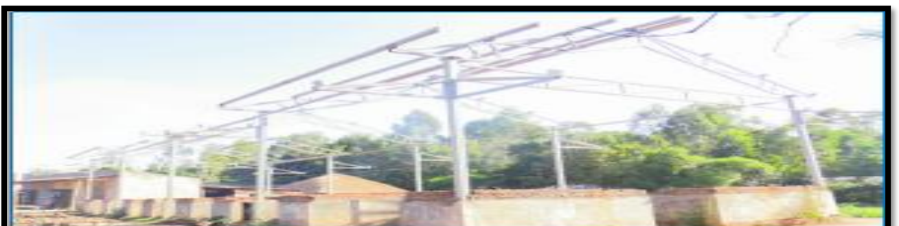
the current status of Siwongo market that stalled since FY 2020/ 2021 and has an allocation of Kshs. 2million for completion of in the approved budget 2023/ 2024
