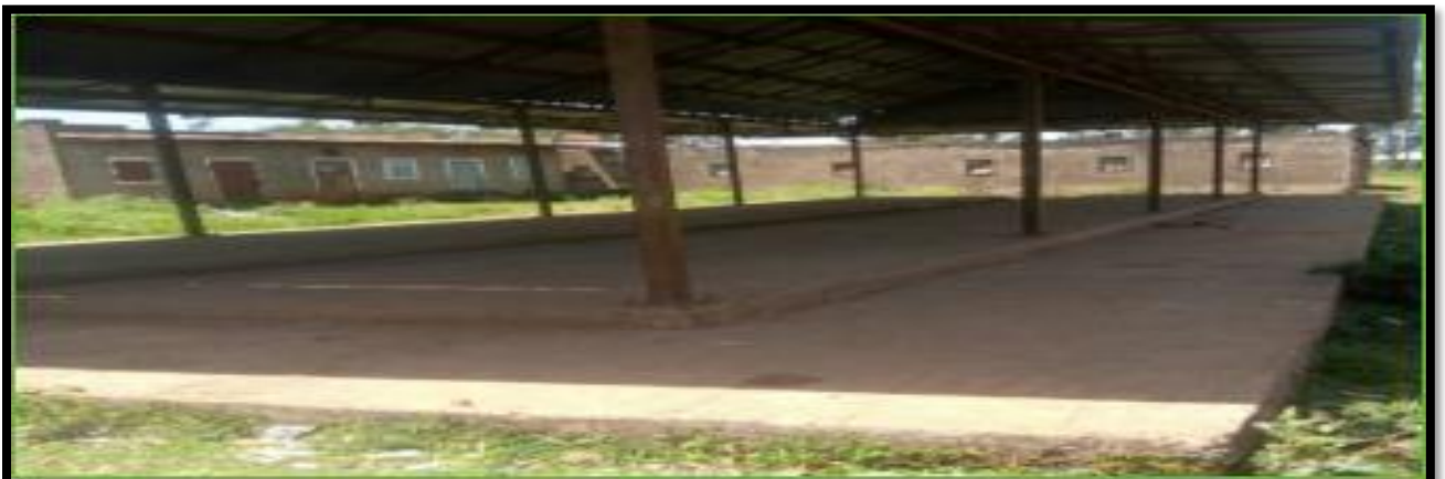
The current status of Bukadanyi market that has stalled since FY 2020/ 2021
